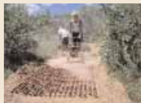
Compacting gravel mixture into Surefoot 4 mats and misting with water for adhesion
